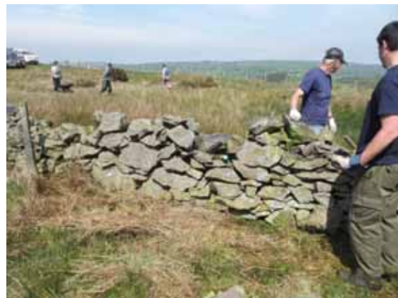
Plate 2: Time ravaged dry stone wall – built from Penstrowed Grit siltstone
