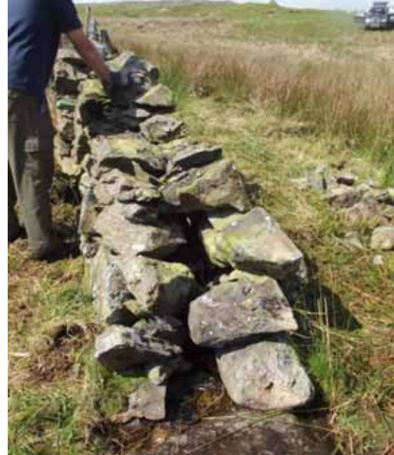
Plate 4: Stripping down reveals loss of “hearting”
